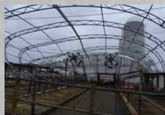
This building was “designed,” just not to the correct loading for the area.
